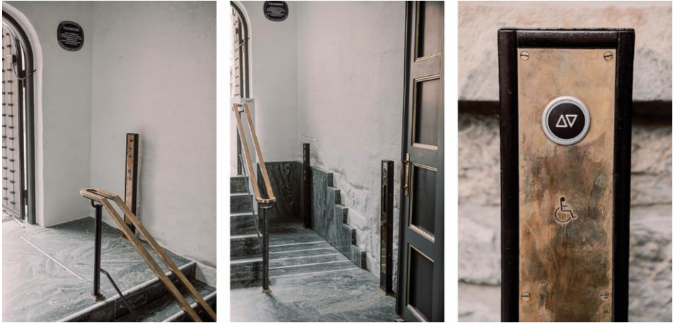
Figure 7. A lifting platform is integrated in the stair in the church's entrance hall. (Photo: Anne-Margrethe Malkenes Mathiesen/The Norwegian Defense Estates Agency)
